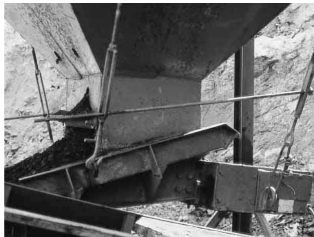
Controlled coal reclaim from an above-ground storage hopper.
